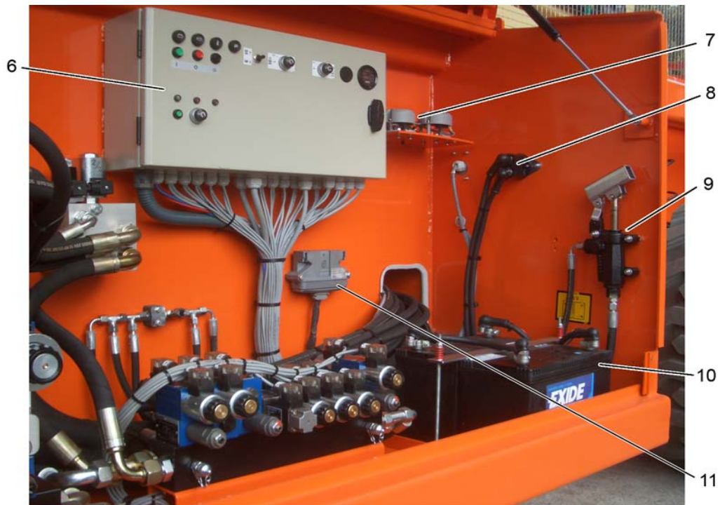
Valves and generator
